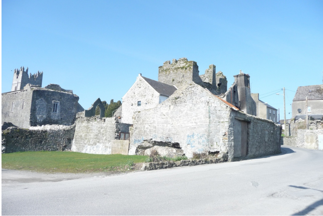
Pic 11. Showing exposed wall at Watergate with evident breach. Note grassed area to fore of wall.
